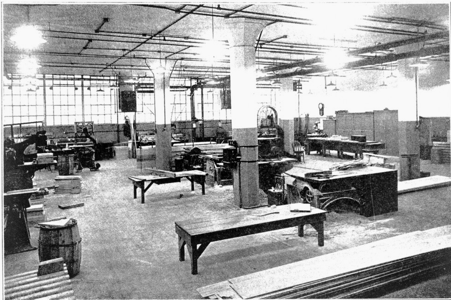
Fig. 44.—An excellent example of modern lighting installation in woodworking shop.
