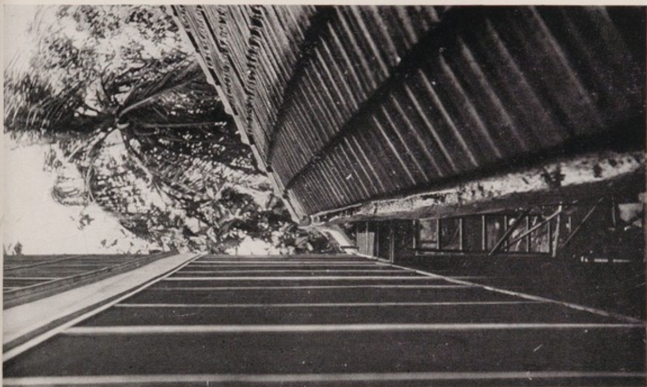
A poorly constructed eave trough
