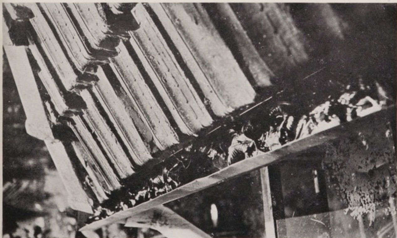
A clogged eave trough
