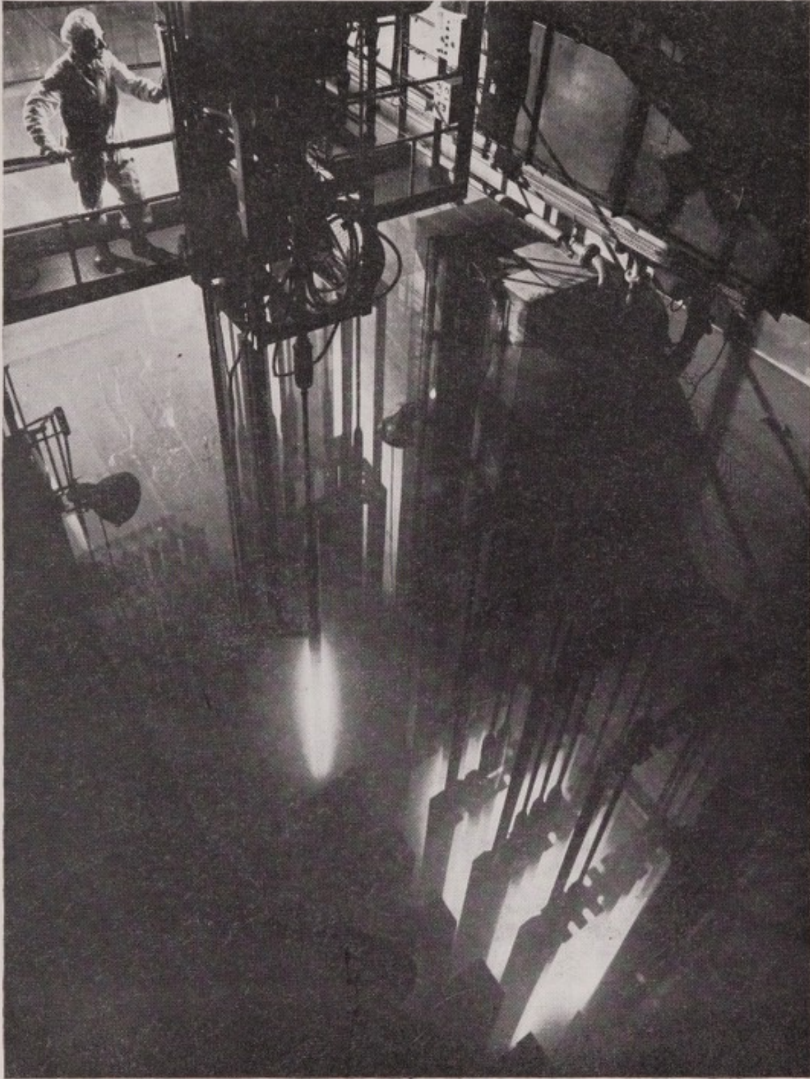
Plate 6. Cooling pond for irradiated fuel elements at the Winfrith 100 MW SGHWR. The 'Cerenkov' radiation surrounding them arises from their \beta -radiation.
