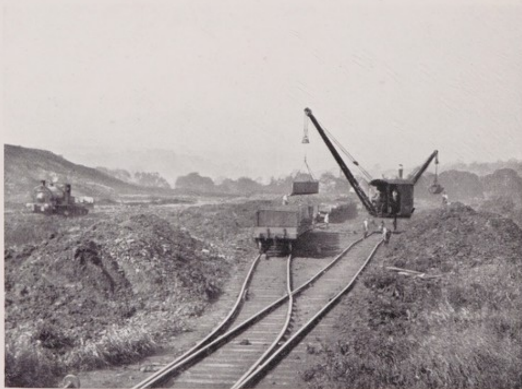
STORAGE AND DRYING GROUND FOR PRESS CAKE.
