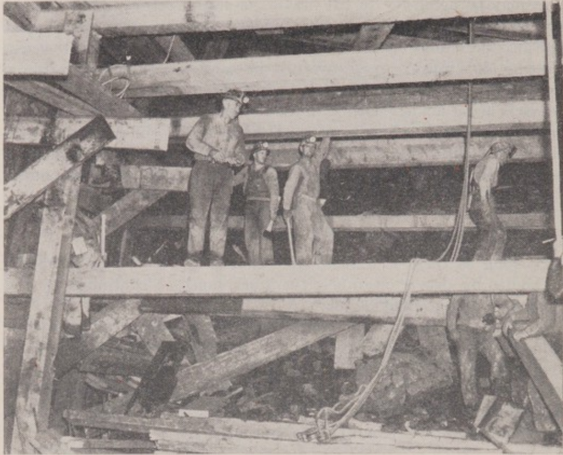
FIGURE 15.—Rescue Squad shoring, bracing, and erecting scaffolding adjacent to pile of debris. Clearance of debris and tunneling work are being done in darkness. Observe rescuers are equipped with individual electric cap lamps, head protection and other standard Rescue Squad equipment. Debris consists largely of timbers, broken concrete and steel members.
