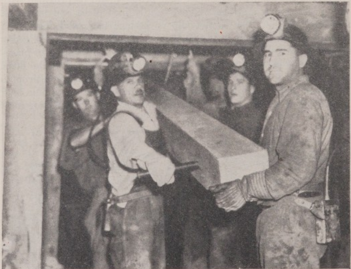
FIGURE 17.—Driving forepoles in a debris tunnel by use of a ram. Three-piece sets, braced at collar, support heavy loose debris.
