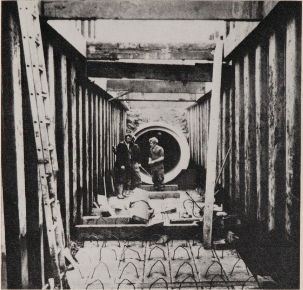
6. A sheet steel piled trench for a concrete sewer on a reinforced concrete bed
