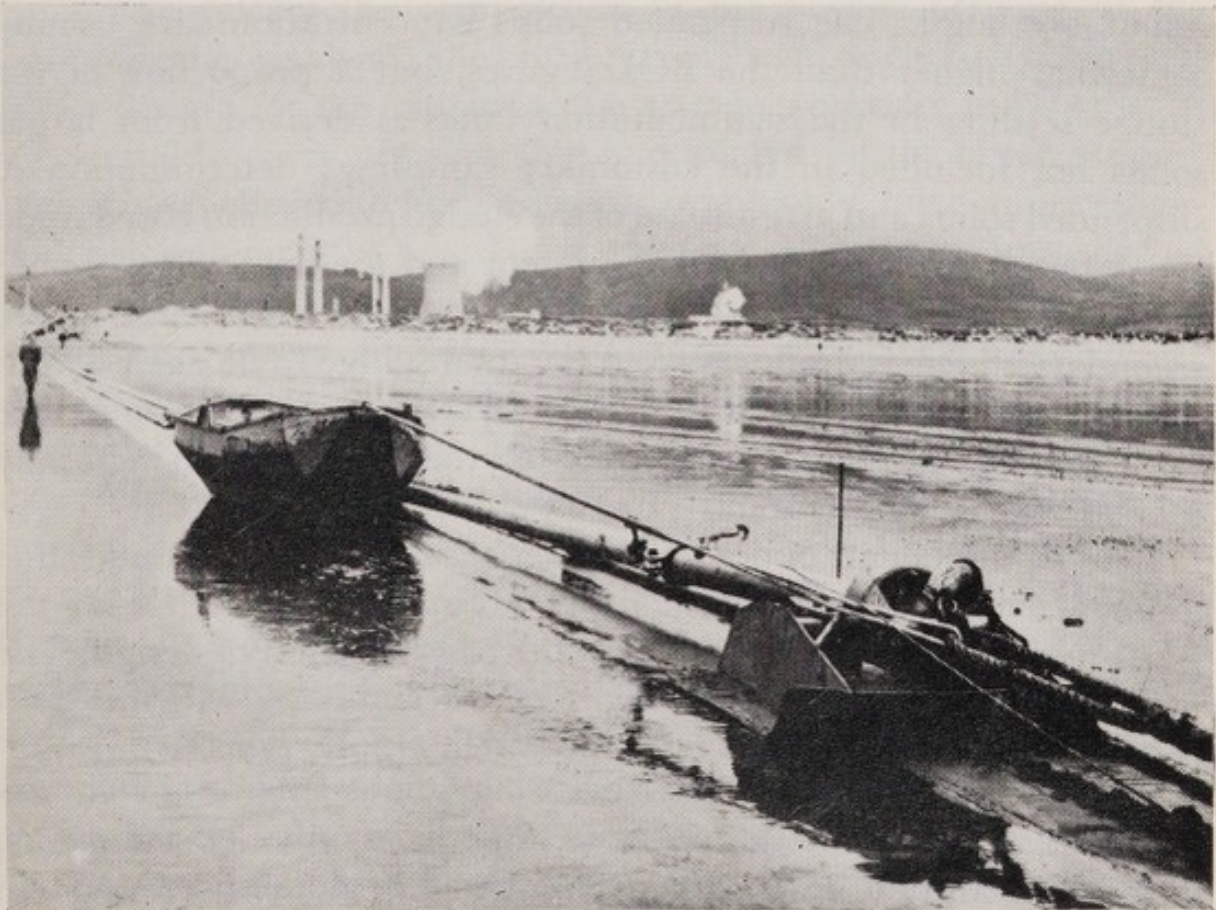
9. A 9840-feet (3000 m) aluminium effluent pipeline for launching into the Severn estuary
