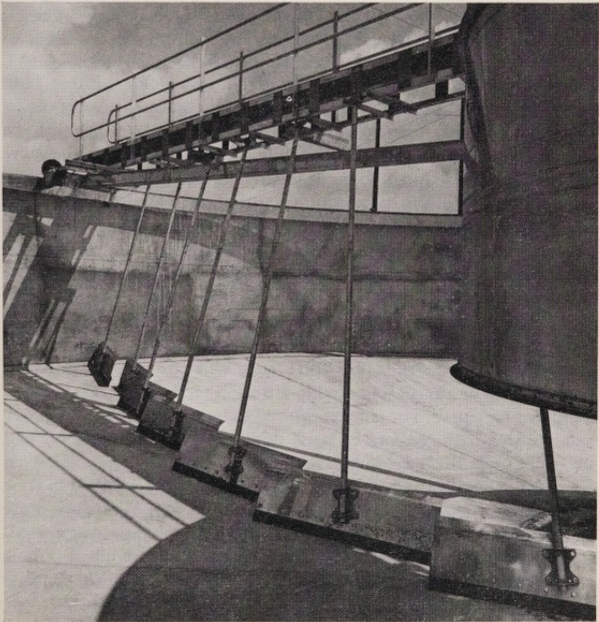
15. Circular tank scraper
