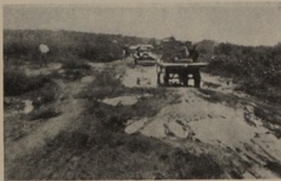
Earth Road broken up by traffic.
