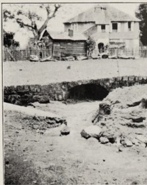
11.—Junction of three drains (note opening of culvert, which runs obliquely under street for long distance).
