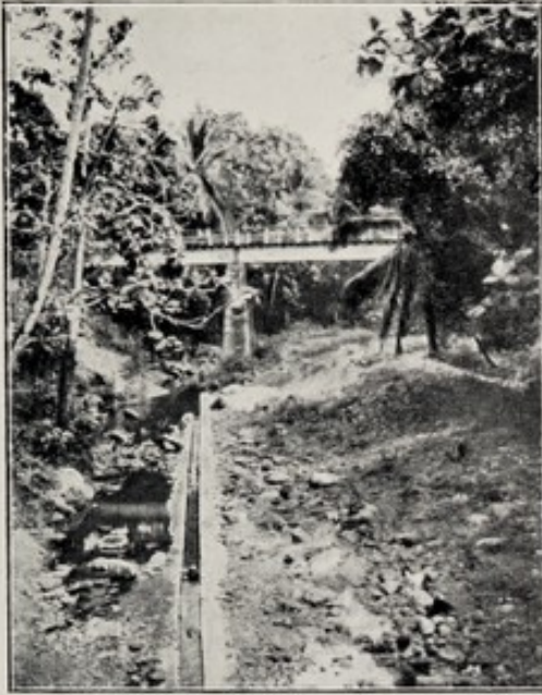
22.—Nicol Brook, canal ineffective through damage by storm flood (dry season).
