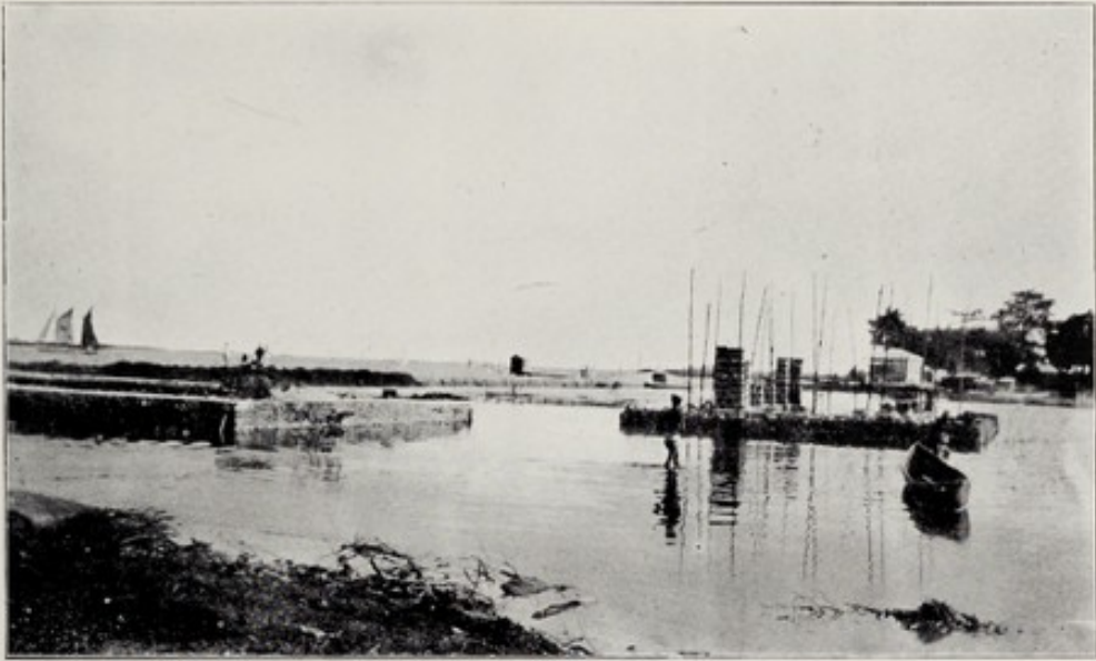
57.—Heddle Swamp, Bonthe, shewing building in swamp (tide full). View from land side looking towards causeway and river. Photo taken late in 1910 shews early stage of house completed in panoramic view taken early in 1911. Note labourer carrying stone wading out to build.
