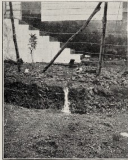
26.—Springs, overflow from under foundations and steps of a Chapel (rainy season).
