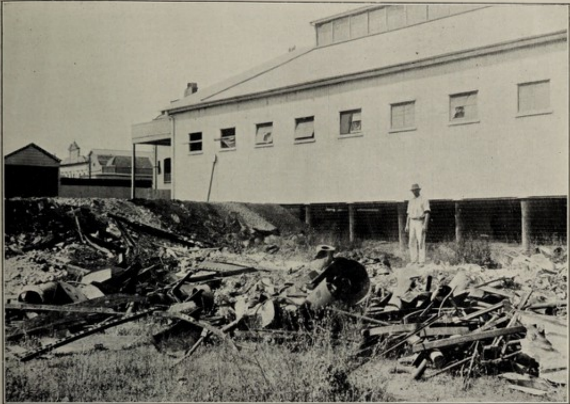
HOW RAT HARBOURAGES ARE FORMED—Vacant allotment being filled in with all manner of rubbish against "K" wire fencing nailed to stumps of adjoining building.
