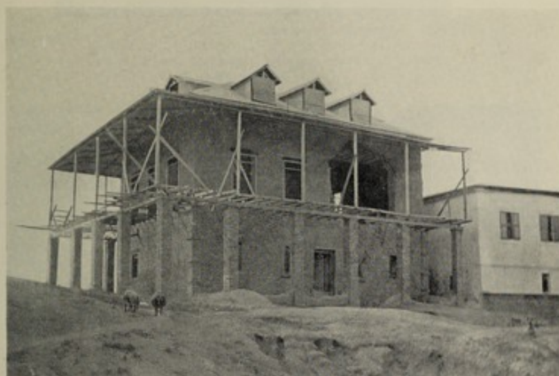
Fig. 2. Acquaye Street. Note large portion of wall fallen in.
