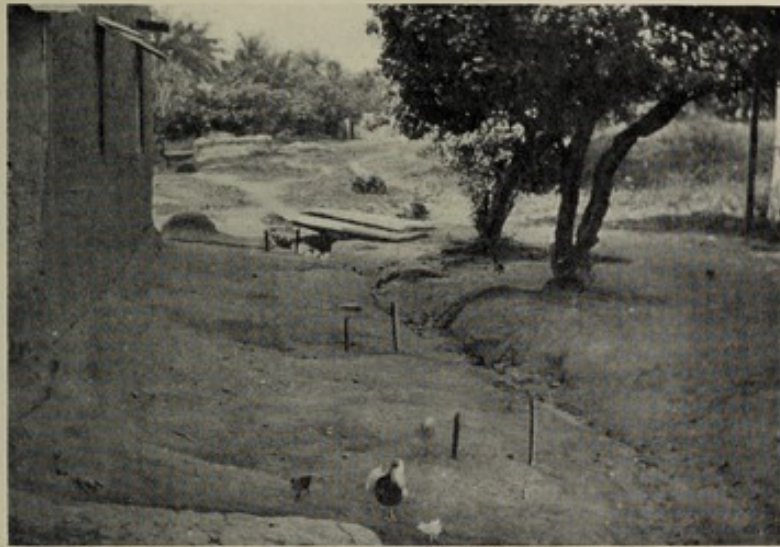
Fig. 11. Water-worn road : Kawanupadu Street. Note planks over natural drain in middle of road.
