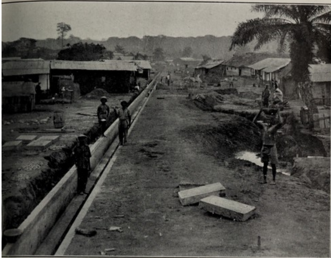
KOFORIDUA. Kano Street drainage. Road before construction.
