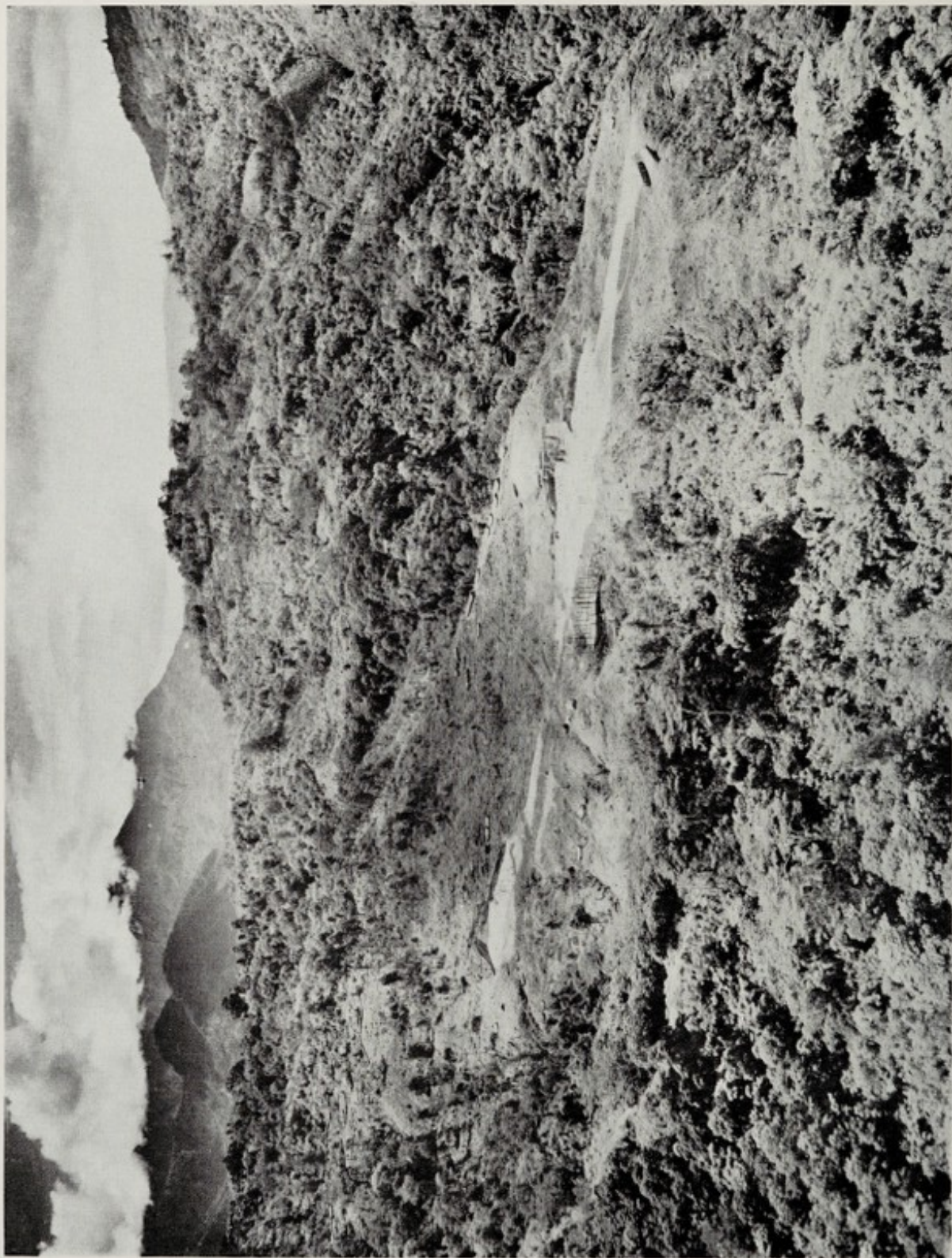
Tabbuga airstrip (altitude 4,300 feet) under construction near the Jimi River Patrol Post in the Western Highlands.
