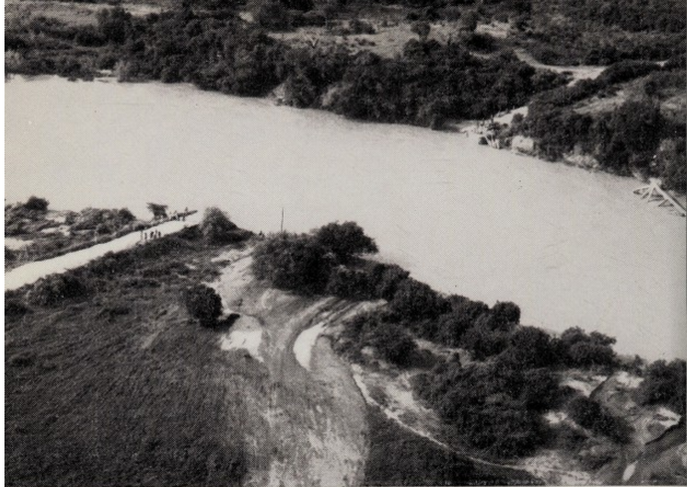
Above. —Aerial view of the Sabaki River, near Malindi, shortly after the road bridge (in water, right) had been carried away
