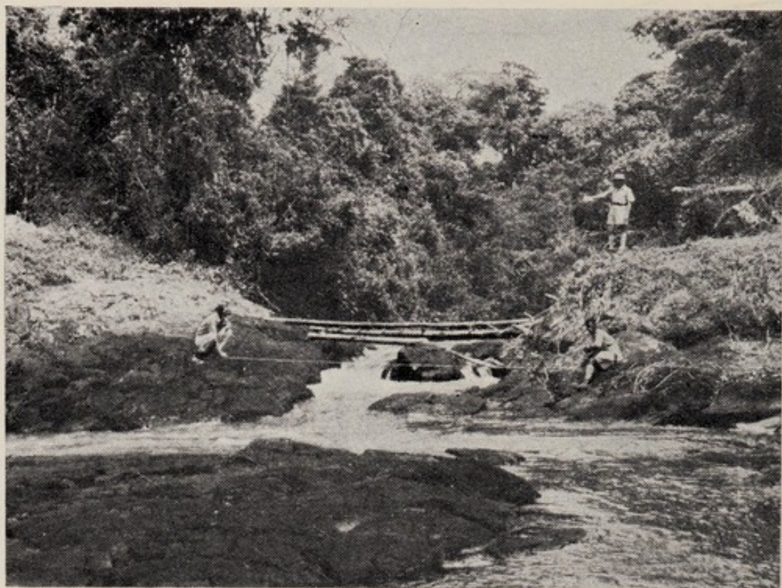
Marking out a site for a new bridge in the Kericho district
