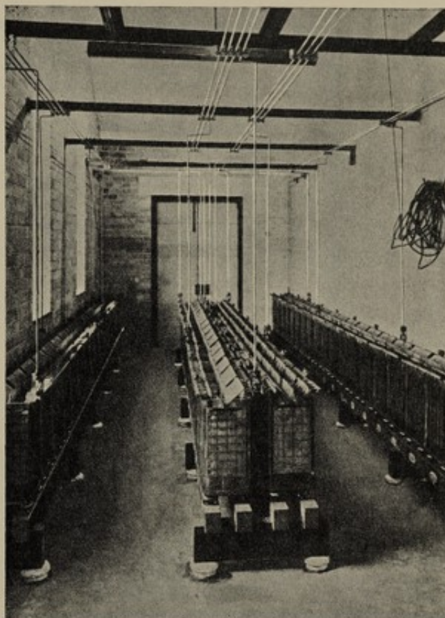
FIG. 41.—Battery Room, Physics Department, University College, Bangor.
