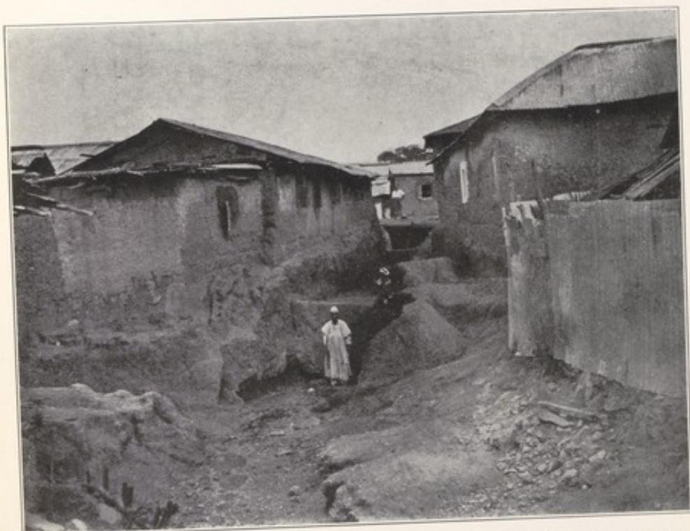
Another street drain showing undermining of house property. Note Inspector standing in drain in background.
