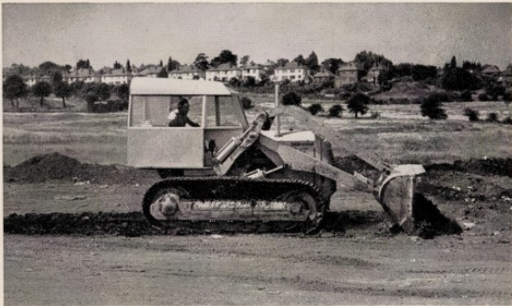
The finished surface is graded to make a good approach road for collection vehicles.
