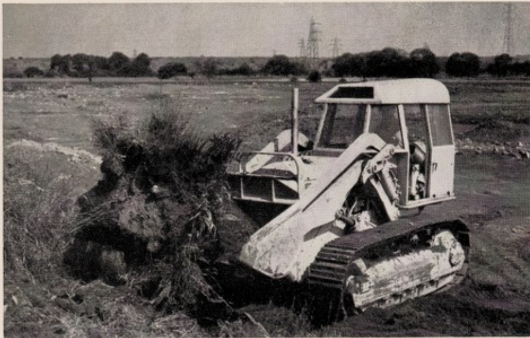
Covering material previously taken off and stored by the HT4 is picked up. It is used to close the tip face.
