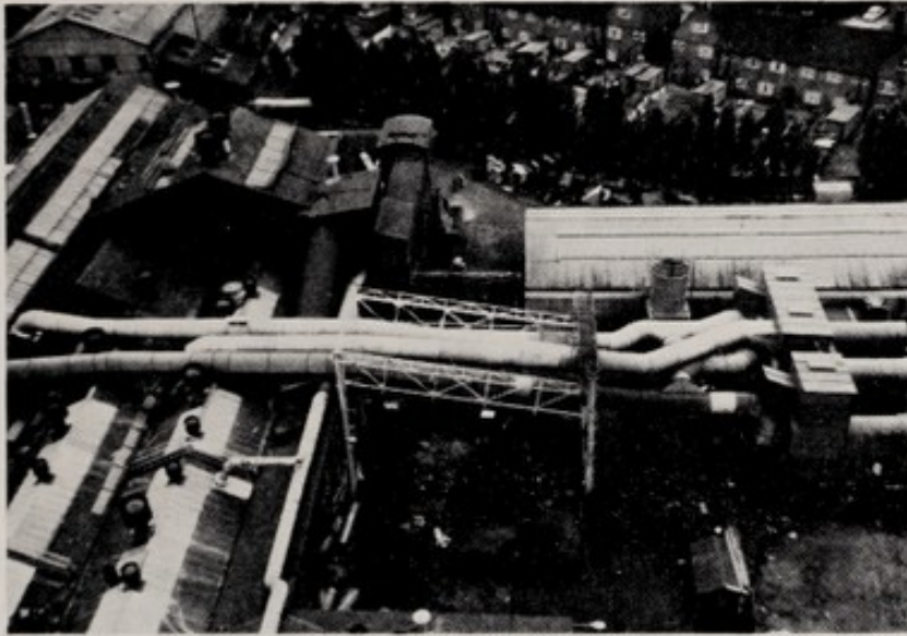
(5) This photograph shows a battery of three wet filters each having a capacity sufficient to deal with 60,000 cubic feet of dust entrained air per minute. The following sources of pollution are included, knock out plant, shot blasting, fettling and grinding plant. The equipment has been acoustically treated to reduce noise levels.
