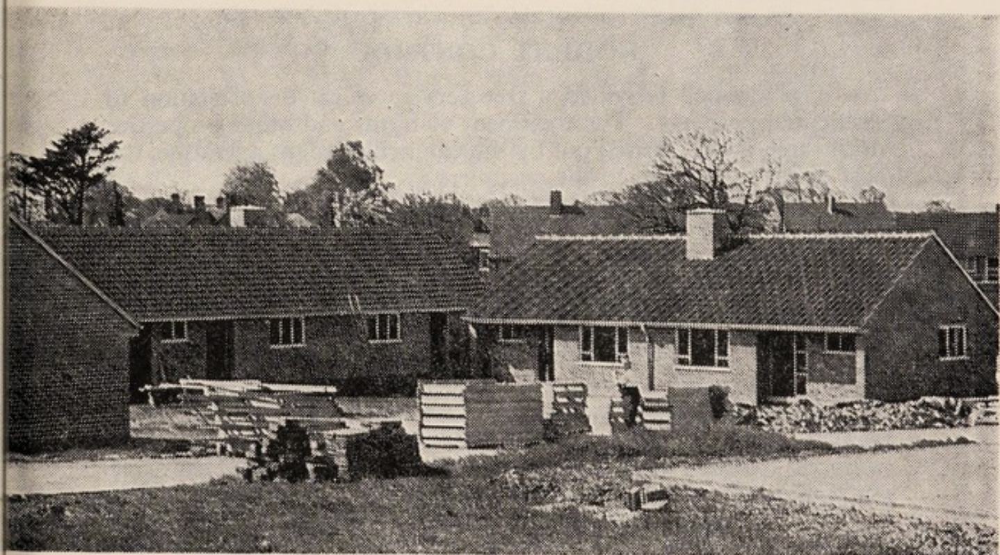
More aged persons' bungalows in course of erection at Wharf Road, Gnosall
