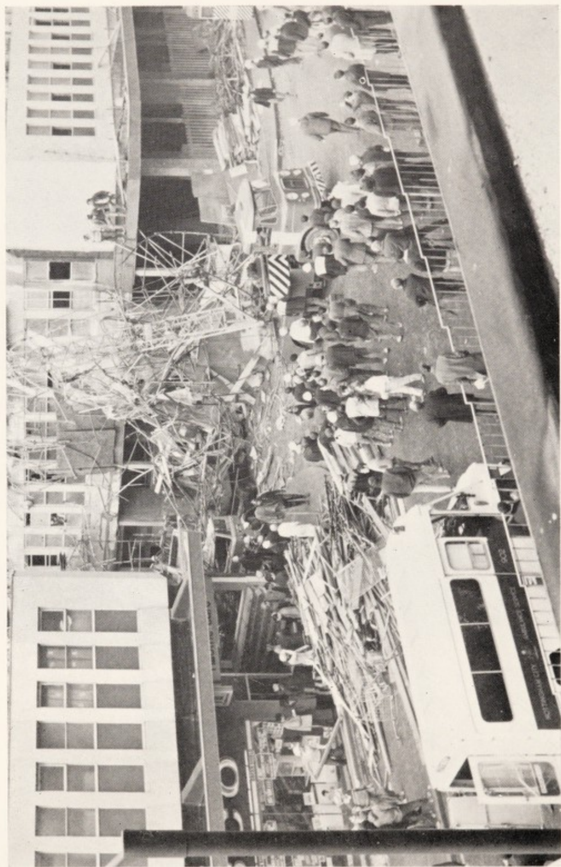
COLLAPSE OF SCAFFOLDING—ALBANY HOTEL
