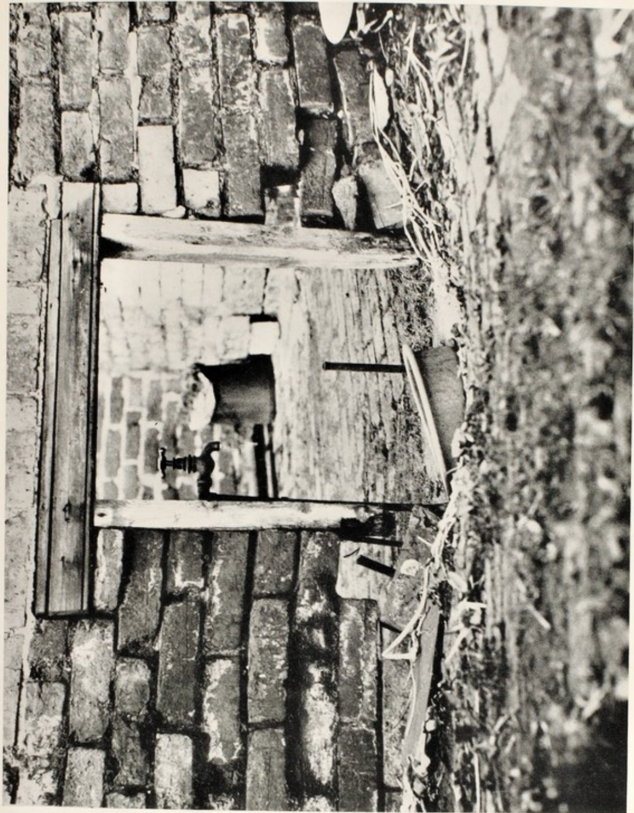
One standpipe shared by two houses and situated in a hole in the yard wall is the only means of water supply to some houses in Northampton.
