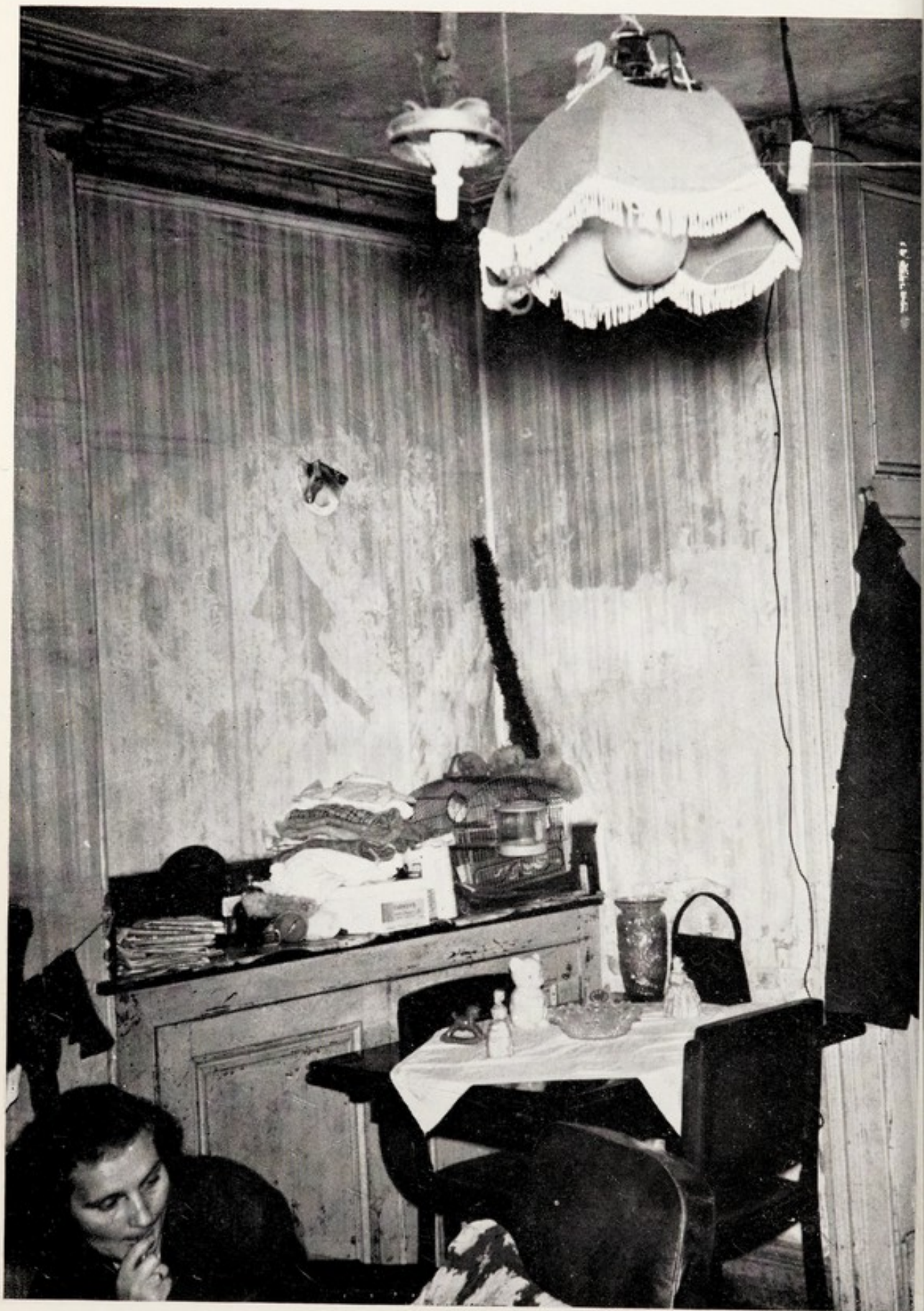
FIG. 2. Extensive rising dampness in walls of only living room.
