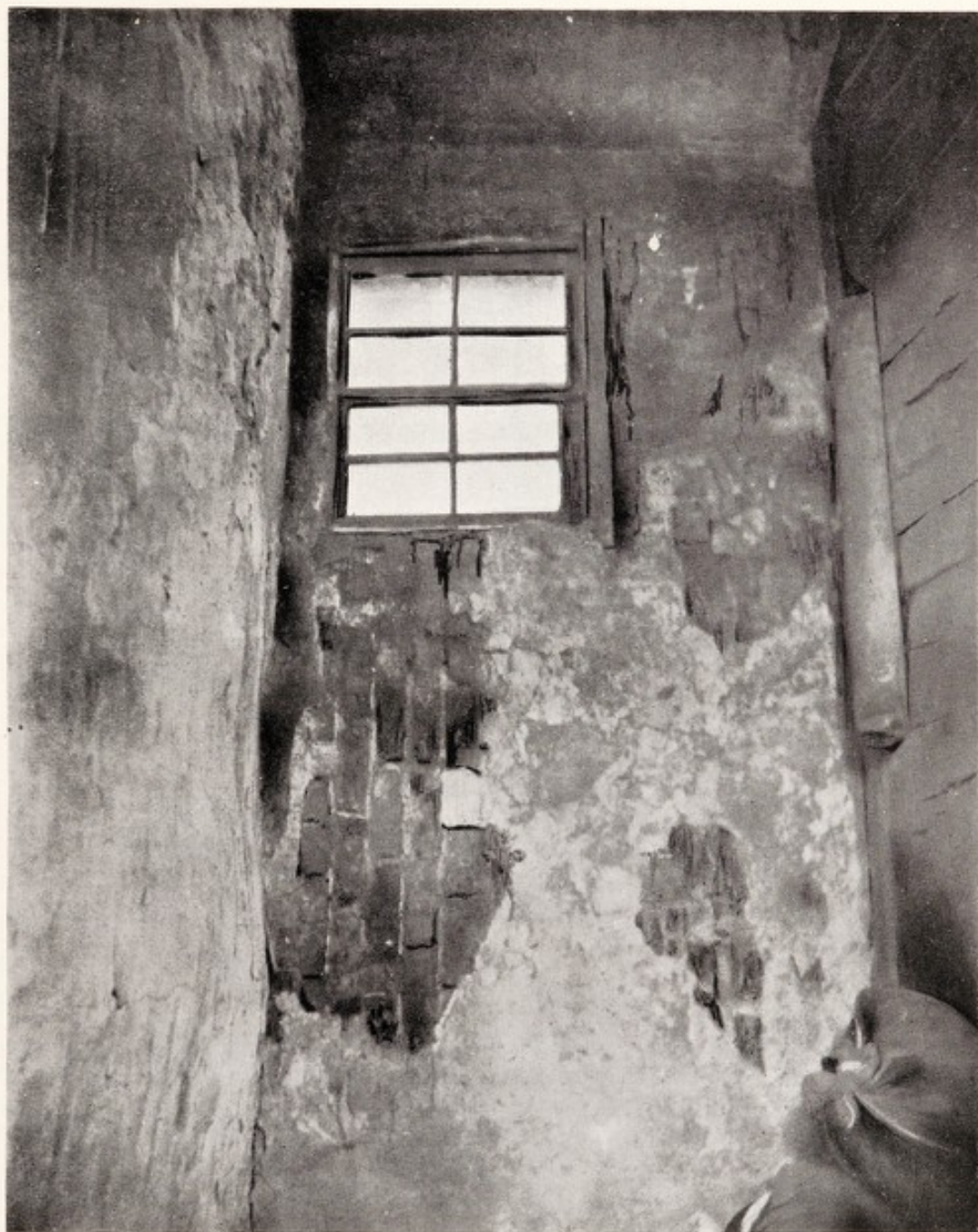
INSANITARY PROPERTY. BEVINGTON STREET AREA.
