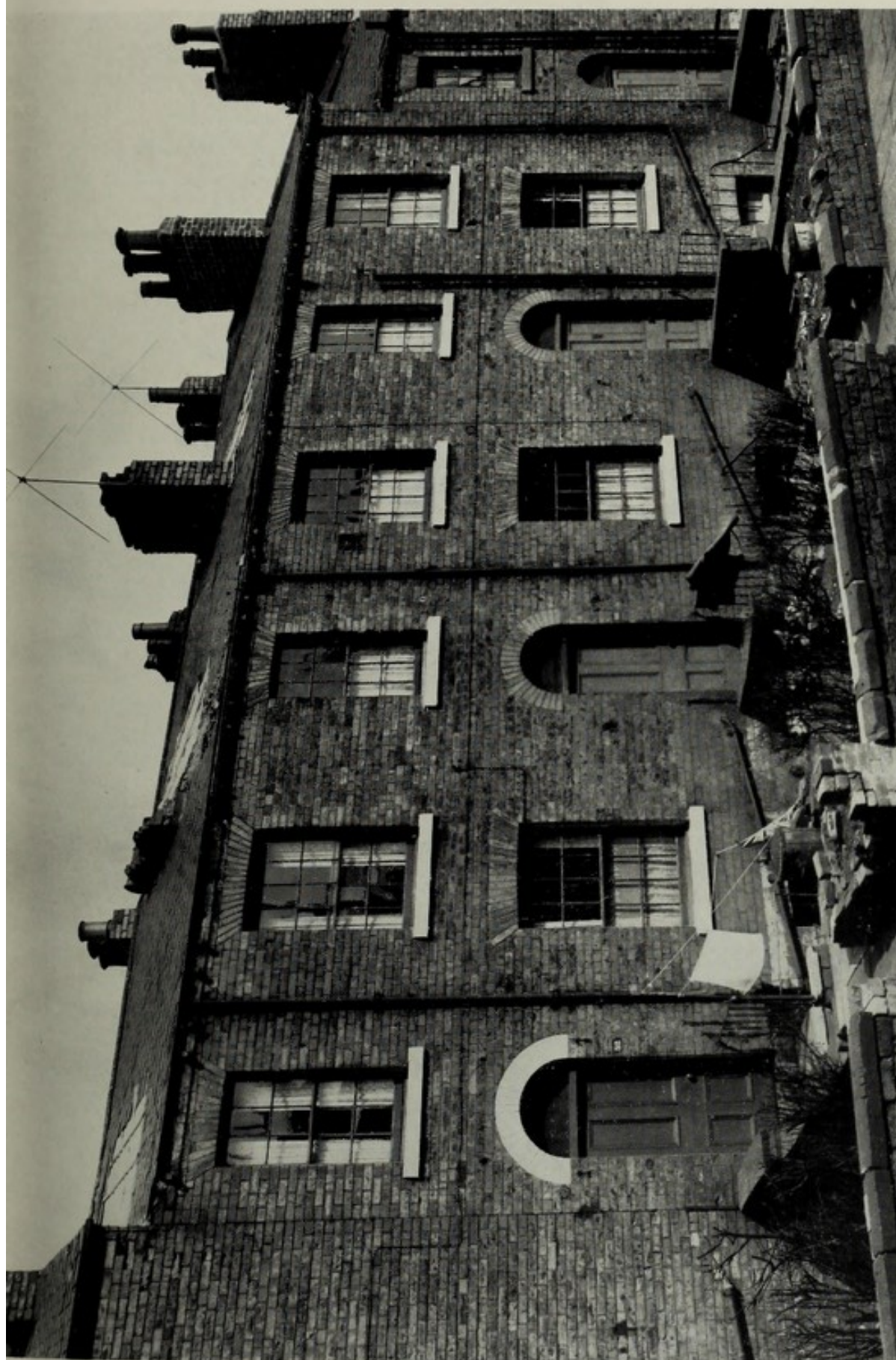
Storm Damage, Nos. 78, 80 and 82, Wallace Street. This block of houses was seriously damaged by the collapse of chimney stacks through roofs causing serious internal damage to the first floor rooms. Closing Orders made by the Housing Committee on 14th May, 1956.
