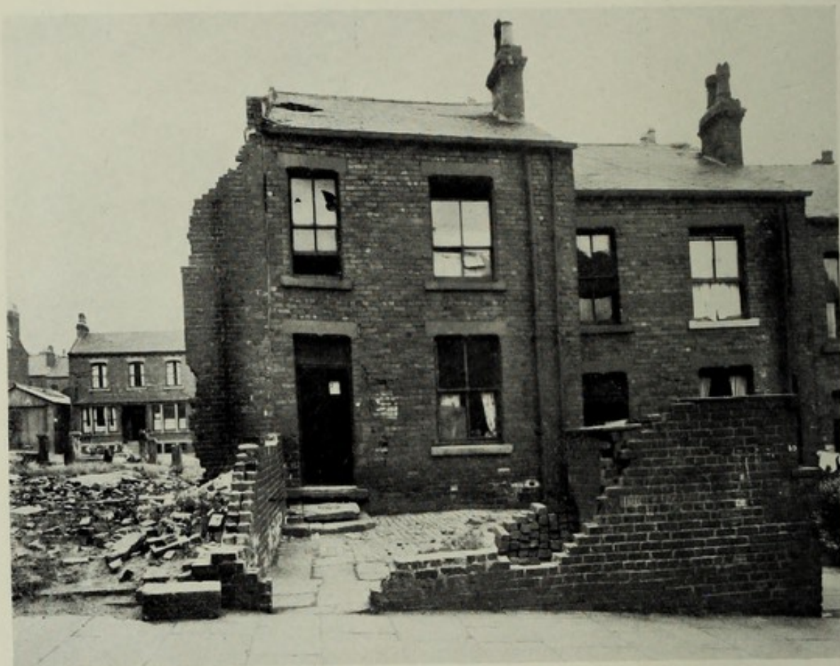
NO. 47, ELMWOOD STREET Showing active danger due to bad settlement. Represented 22nd October, 1948, demolished 12th July, 1949.
