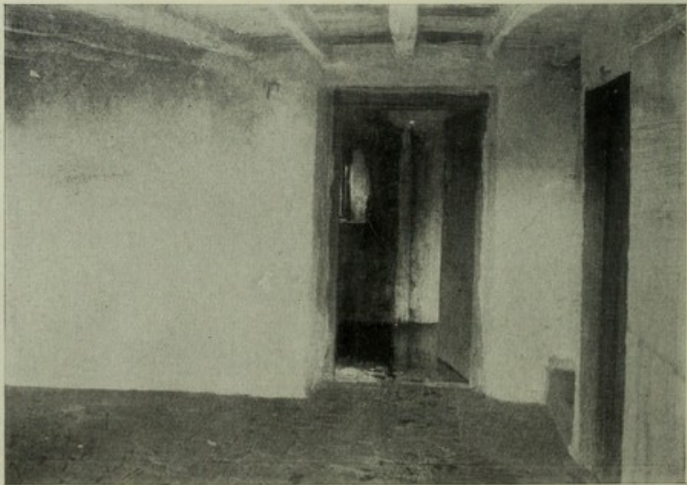
No. 4. Shows a view of the interior of the "Hospital." The construction of the floor of the front room is clearly shown. Although at the time the photograph was taken there had been no rain for a month, water stands several inches deep on the floor of the back room seen through the doorway. There is no furniture.
