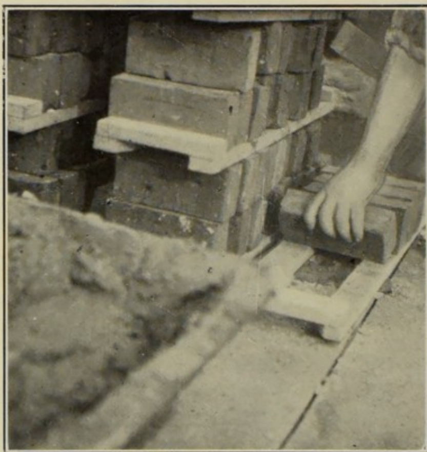
Fig. 7. — Wrong way to pick up brick from the lower tier on the packet.
