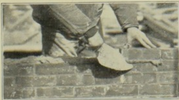
Fig. 38.—Working left to right.—Cutting off mortar after brick is laid on exterior face tier.
