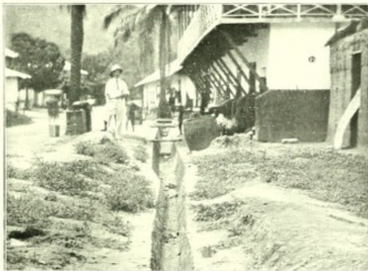
Surface drain at Dodowah, showing bad construction.
