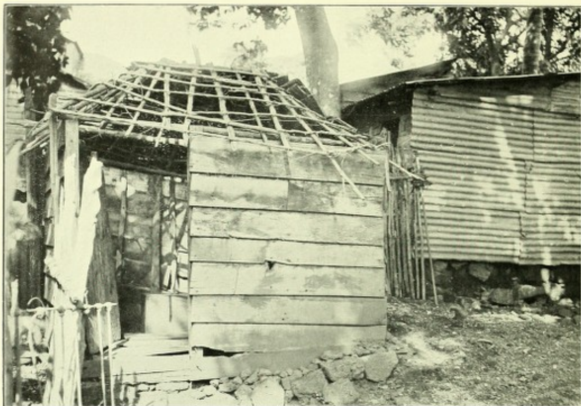
Dilapidated cesspit behind house, showing partly denuded rafters on roof, loose rubble coping, broken walls and floor, next to it a corrugated iron shelter over a cesspit with defective coping. [See page 30.]
