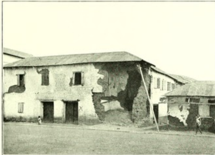
Dilapidated houses in principal street.
