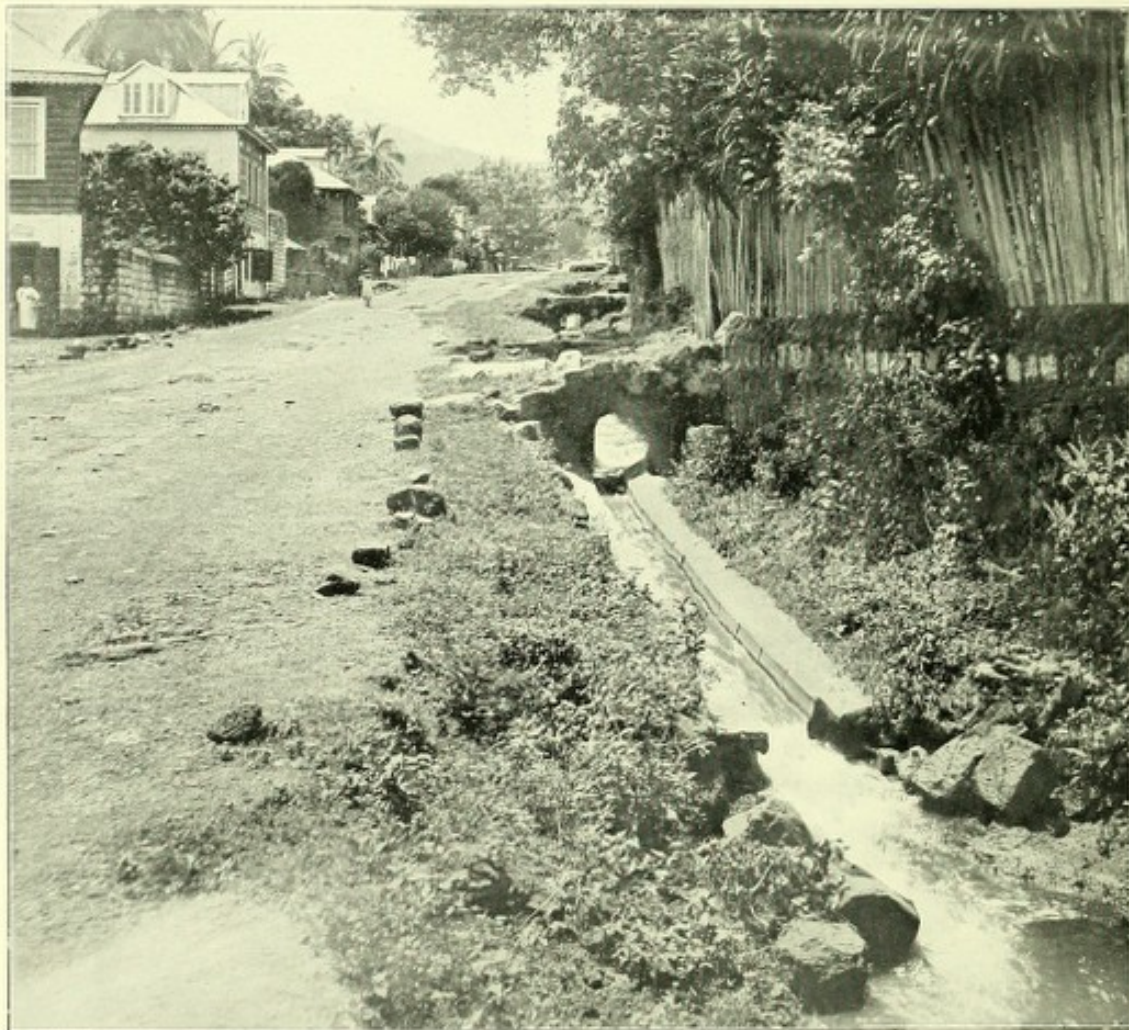
Street drain. Circular Road at junction with Regent Road, showing water spread over bottom flat square drain passing the smooth semicircular 12 in. half-pipe drain and only half filling it.
