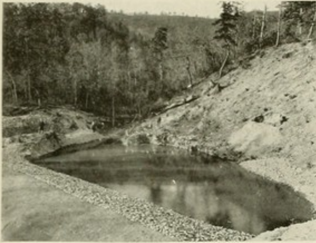
No. 17.—Catawba Sanatorium, Catawba, Va. AN EXAMPLE OF A GOOD METHOD OF STORING WATER WHERE STREAMS CAN BE PROTECTED FROM CONTAMINATION. (See illustrations 30, 69, and 80 for further description of this institu- tion.)
