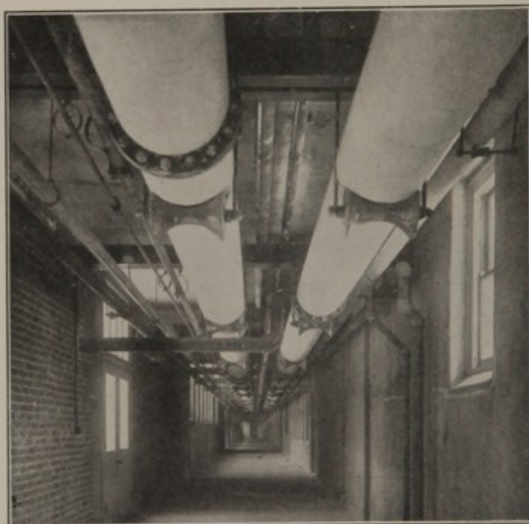
Fig. 15.—View of main tunnel near power plant. (Note large size of hot-water pipes.)
