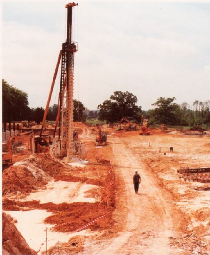
LEFT: Builders first dug a huge hole to accommodate the underground car park.
