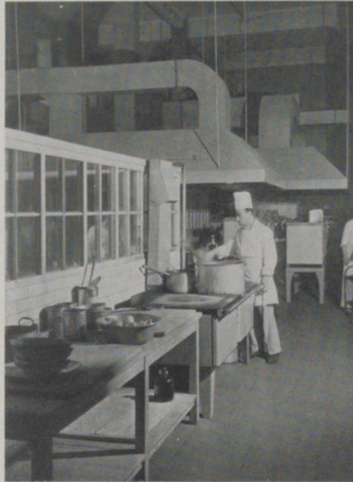
Central gas cooking stoves with canopies and extractor fans
