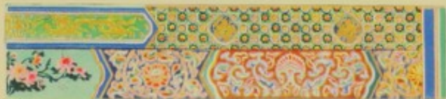
Detail of beam in the East Covered Walk of the Fu Jih Lou.
