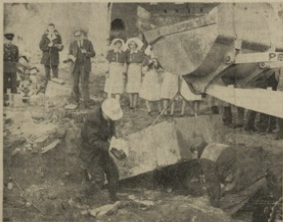
The 21-ton Welsh granite foundation stone is gently lifted from its 119 years old resting place.
