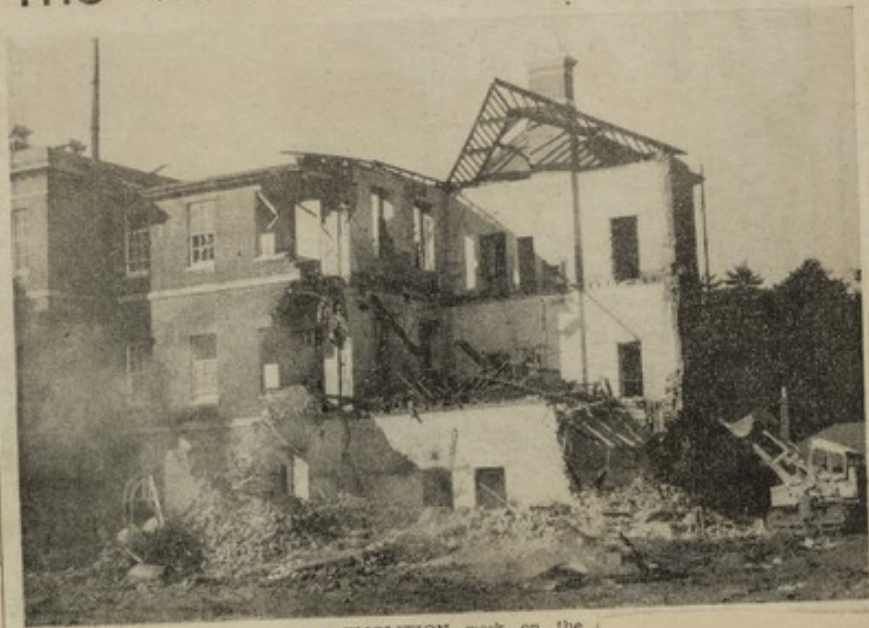
D EMOLITION work on the west wing of the Royal Victoria Hospital at Netley is well under way although most of the building is still intact.— Photo: A. McIntyre.
