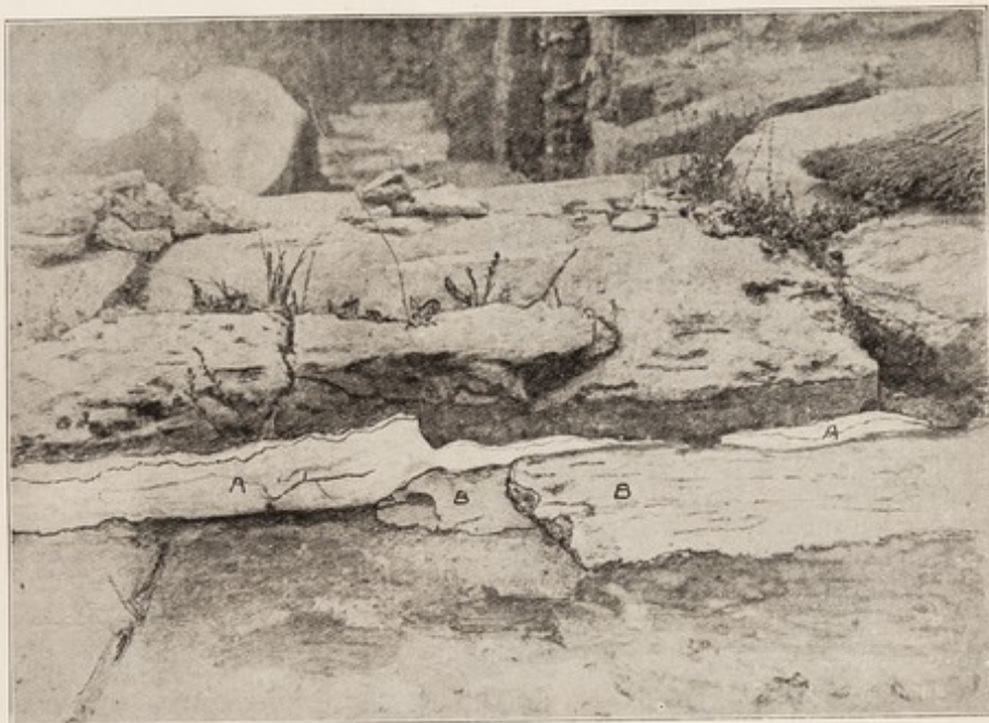
FIG. 12.—FOUNDATIONS OF THE WEST WALL, CENTRAL COURT, KNOSSOS, SHOWING THE PLASTER (A) BENEATH THE CEMENT FILLET (B).
