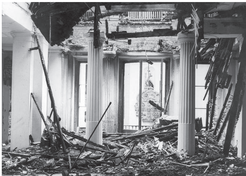
Figure 15. The inner hall of the Royal College of Surgeons of England (See Fig. 17) damaged by the Blitz on 11 May 1941, photograph late May 1941. The rebuilt college was opened, formally, by Her Majesty Queen Elizabeth II, accompanied by The Duke of Edinburgh, on 7 November 1962.
